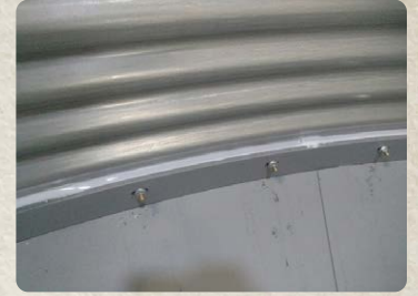
Inside bin bolted to hopper
